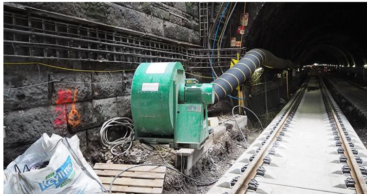
Ventilation Queen Street Rail Tunnel, Glasgow
